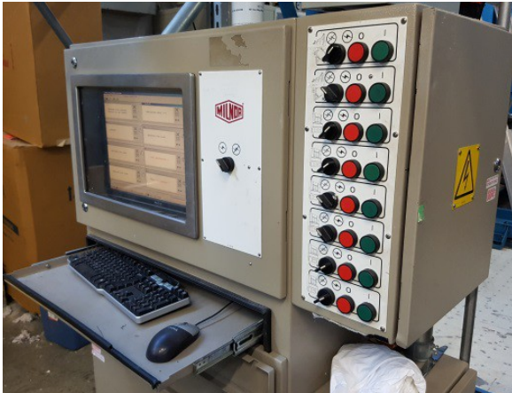
Dryer Row 1 Control
